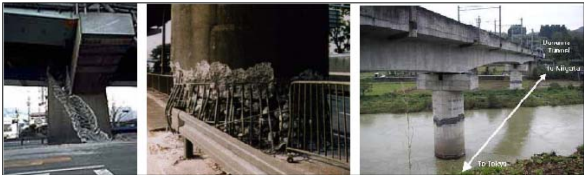
a) Shear failure
