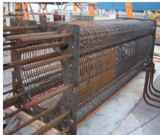
(d) Use templates at both ends of the cages to position the main bars.
